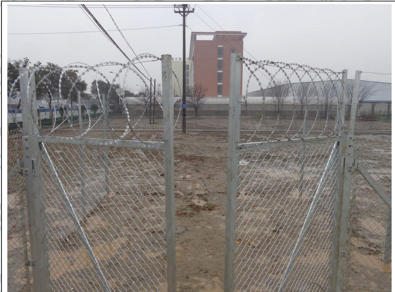
65). Start laying the razor wire on top of the tensioned wire, attached with pieces of tension wire. It is much faster if you have two persons working together, one on the inside of the fence and the other on the outside. Continue with the same process to cover the entire fence length
