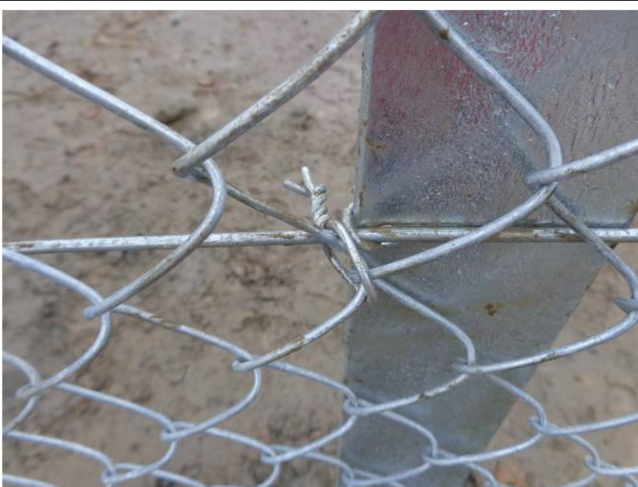
49). View from Outside the fence. A typical way of connecting the chain-link mesh to the tension wire
