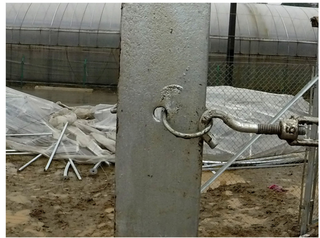
29). Connect the tensioners to the razor wire support as described here or in (Pic.28)
