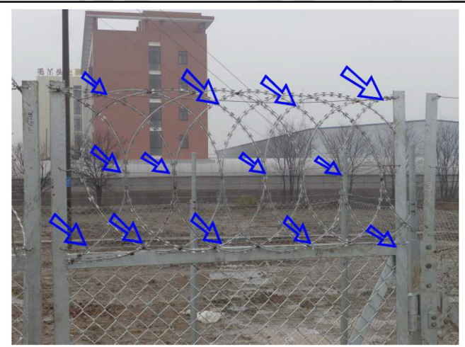
67). Connect the flat wrap type razor wire to the tensioned wire in several locations as described.
