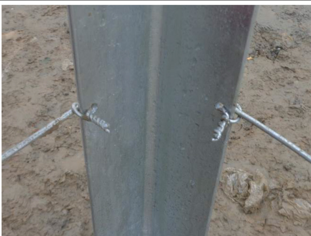
36). Tighten the small pieces of wire after all tensioners are tightened (View from inside)
