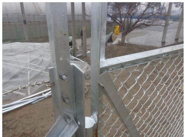
77). Inside view of gate post &amp; razor wire support
