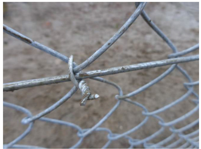
46). View from inside the fence. A typical way of connecting the chain-link mesh to the tension wire.
