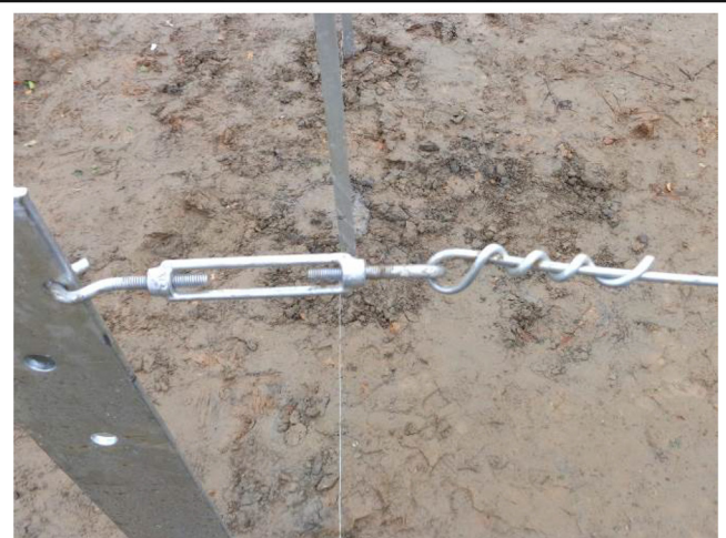
25). Connect the tension wire to the tensioners as described here or in a similar way
