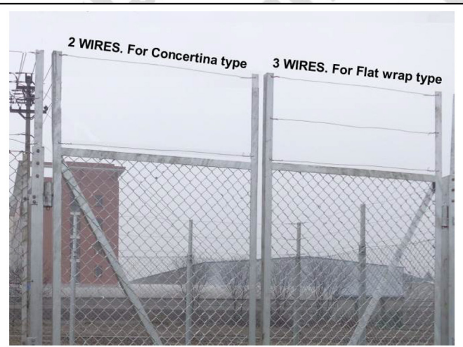
64). Tension wires installed as described earlier. Quantity depends on type of razor wire product type.
