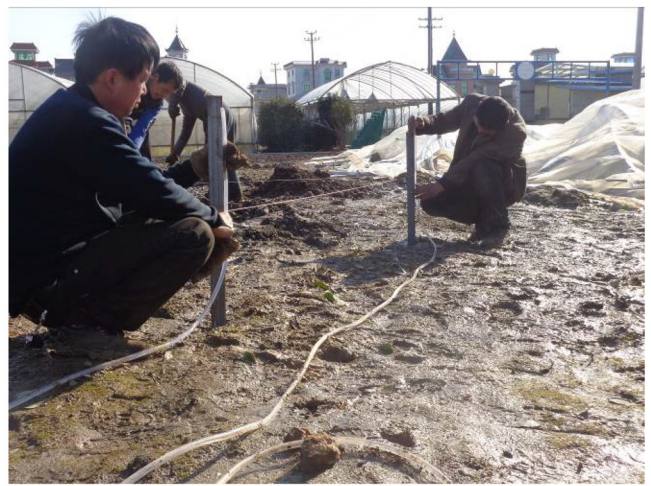
02). Place the first two spikes and identify the frontal section of the fence, face "C" to "D".
