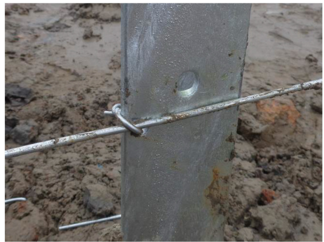
35). Tighten the small pieces of wire after all tensioners are tightened (View from outside)
