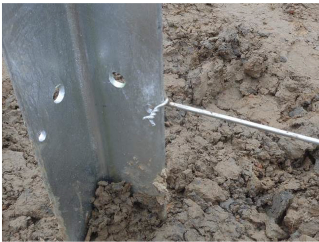
34). Tighten the small pieces of wire after all tensioners are tightened (View from inside)
