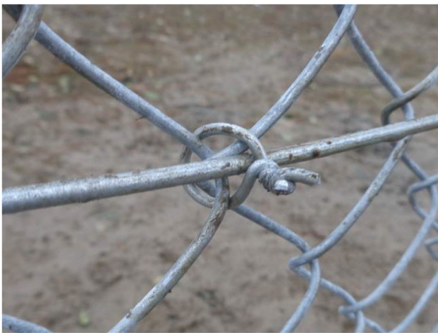
47). View from inside the fence. A typical way of connecting the chain-link mesh to the tension wire.
