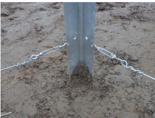
30). View from inside of tension wires and tensioners.
