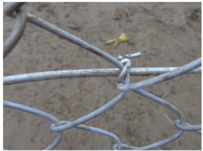
48). View from Outside the fence. A typical way of connecting the chain-link mesh to the tension wire
