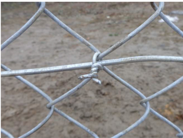
45). View from inside the fence. A typical way of connecting the chain-link mesh to the tension wire.
