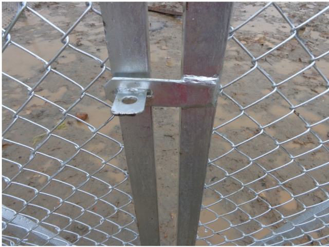
20). The gate is locked by a hasp and staple as indicated here.
