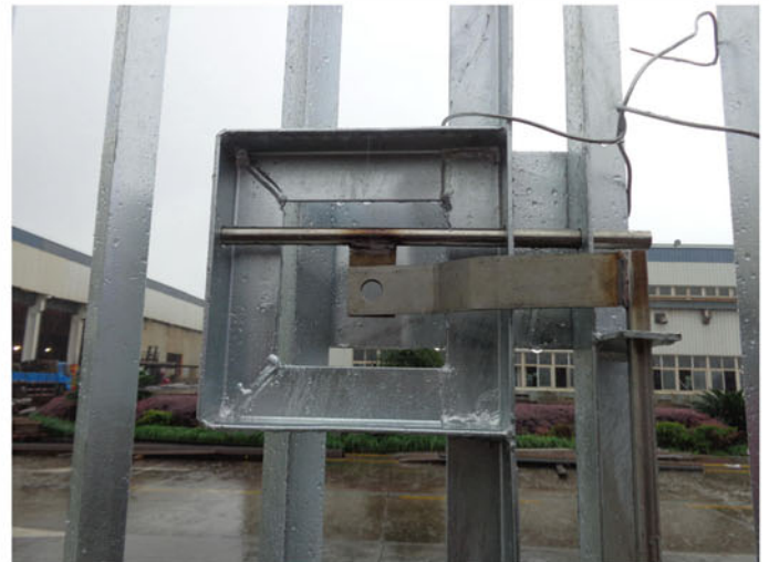
Trial of Palisade fence – stainless steel lock (Note that at this stage pales are installed facing inwards to avoid using original locking bolts)
