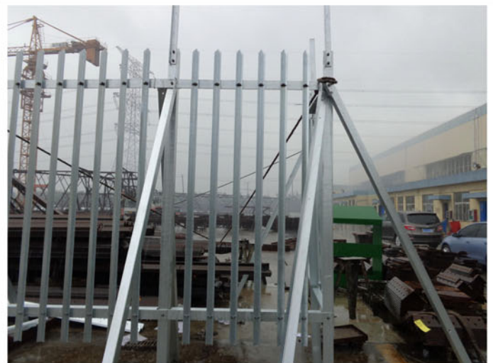
Trial of Palisade fence – 1200mm panel (Note that at this stage pales are installed facing inwards to avoid using original locking bolts)
