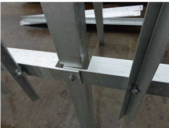
Trial of Palisade fence – Horizontal supports (Note that at this stage pales are installed facing inwards to avoid using original locking bolts)
