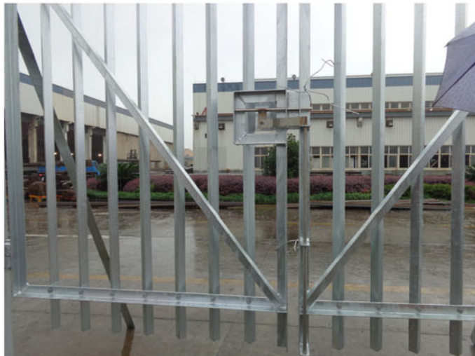
Trial of Palisade fence (Note that at this stage pales are installed facing inwards to avoid using original locking bolts)
