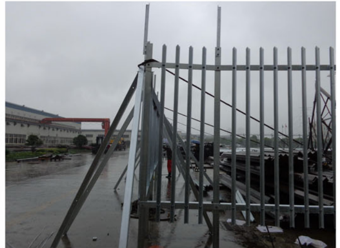
Trial of Palisade fence – 825mm panel (Note that at this stage pales are installed facing inwards to avoid using original locking bolts)
